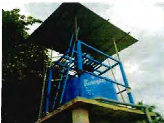
FOTO 55: Reservoir of the JASS-LAS BALSAS, equipped with a chlorination system, infrastructure of metal for the protection of the tanks dispensing the water service and roof. The system is complete and operational.
